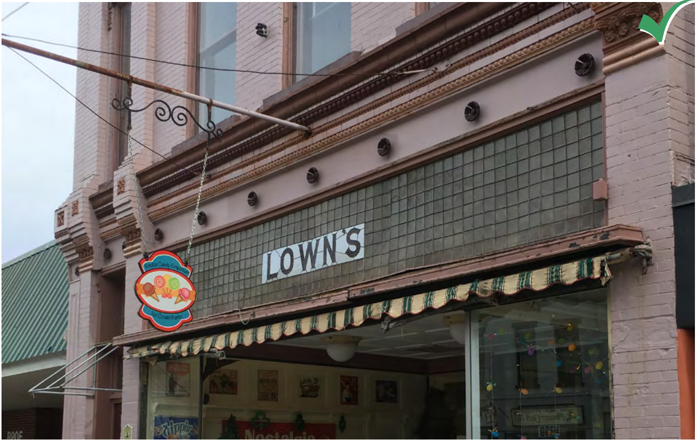
Restore and maintain historic leaded glass transom windows, cornices, and masonry detailing when possible.
