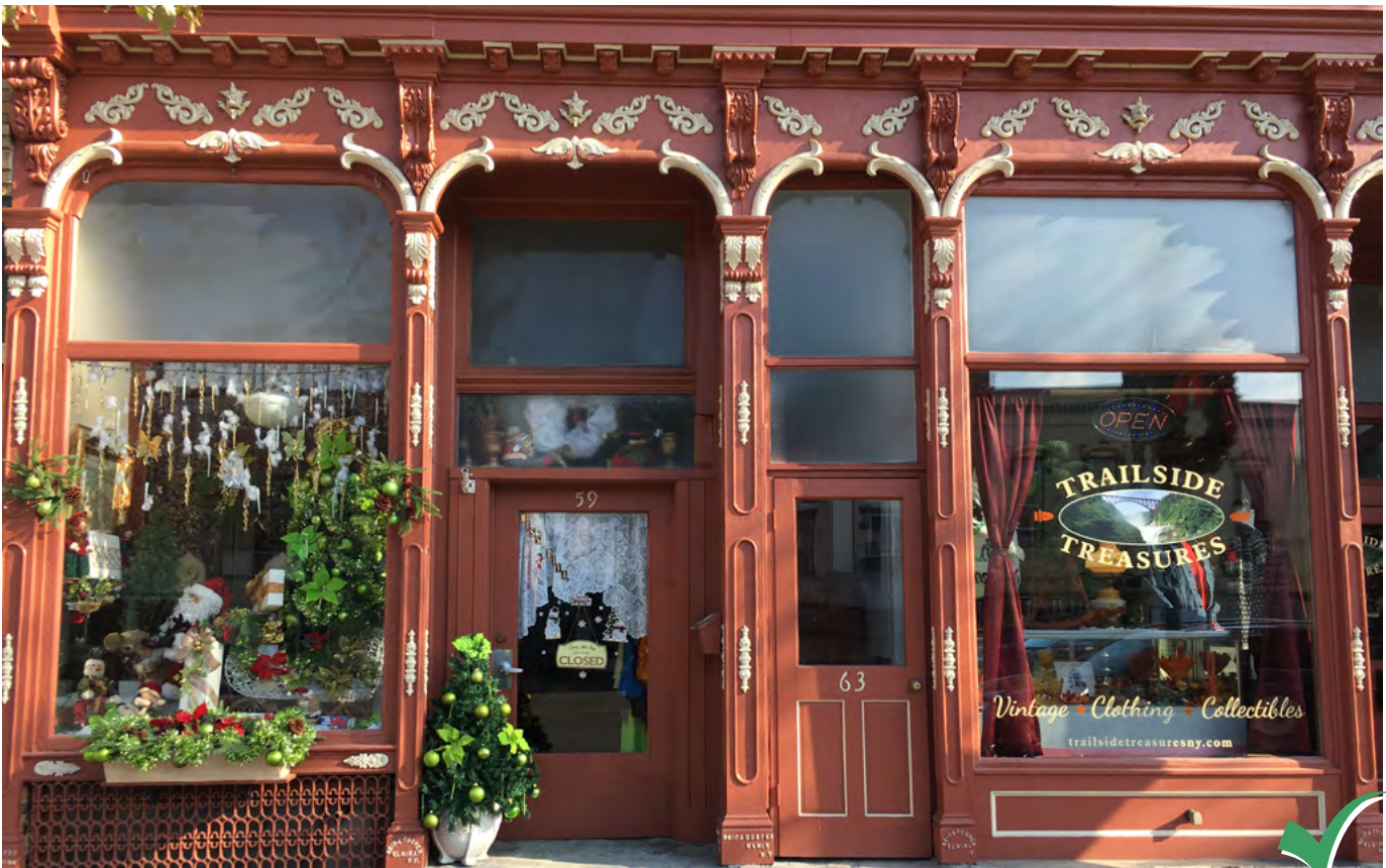
Original steel columns and cornices can be uncovered and restored to provide authentic character to a storefront.
